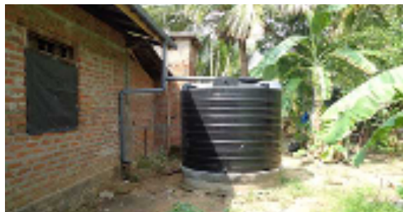
Figure 10: Rainwater harvesting tank
