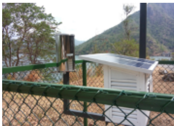
Figure 8: Automatic rain gauge installed in Walapane
